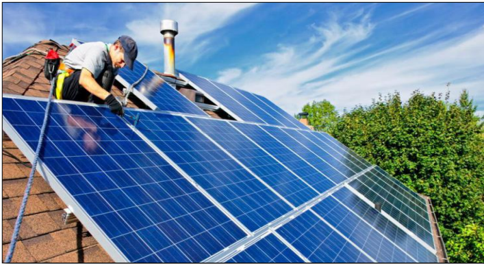
Courtesy: Rob Stubbins Solar Energy
